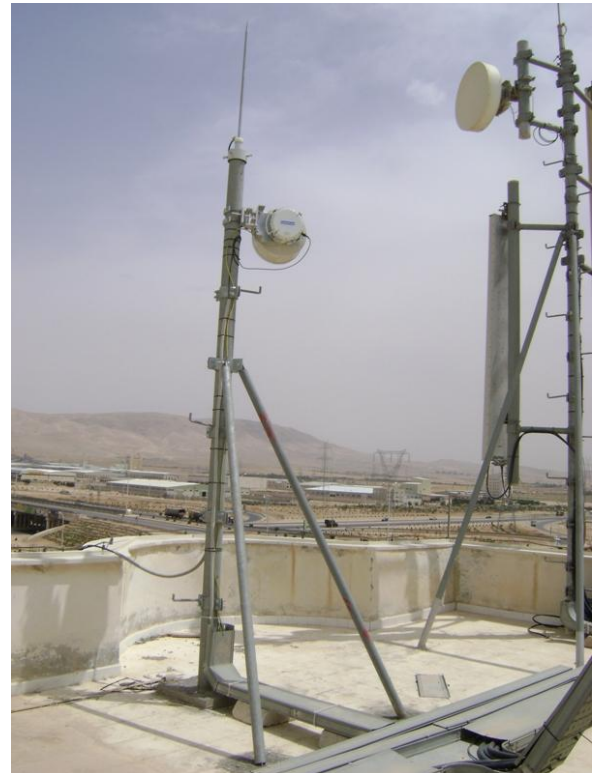
CableFree Microwave Backhaul links installed in the Middle East
