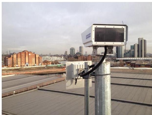
CableFree UNITY installation in London, combines FSO + MIMO Radio for Resilient, Diverse Media, 1+1, zero single point of failure, ultra-high-availability networking
