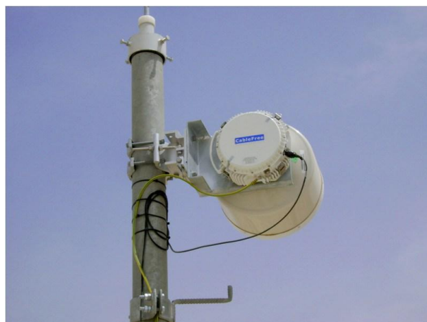
Installation of CableFree Microwave Link takes a few hours, compared to days or weeks for cable/fibre digs.
